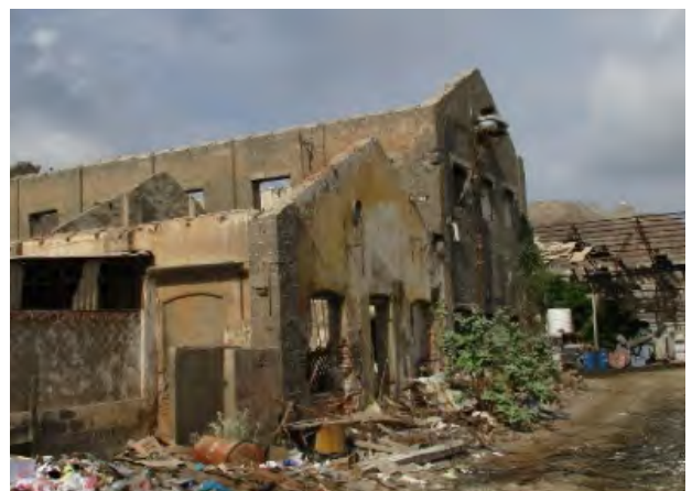
State of Power House in Al Mualla (UNESCO 2019)
